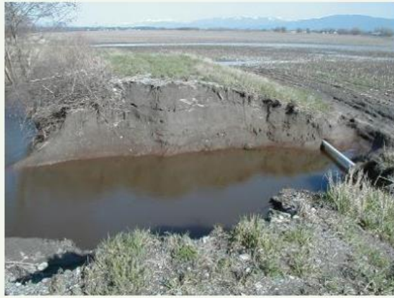
Reach 2 Levee Breach
